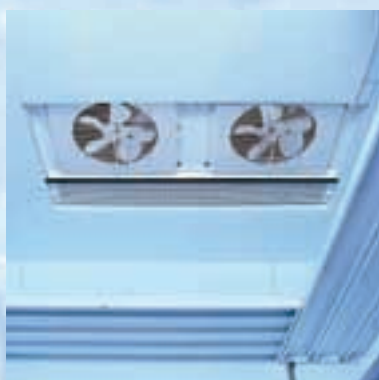
Powerfull evaporator fans circulate the air on the roof top freezer unit.
